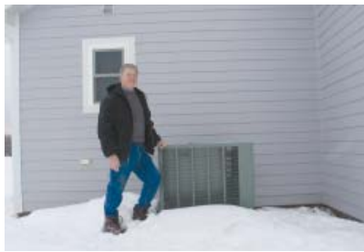
John Beatty installed this 17 S.E.E.R. heat pump.
